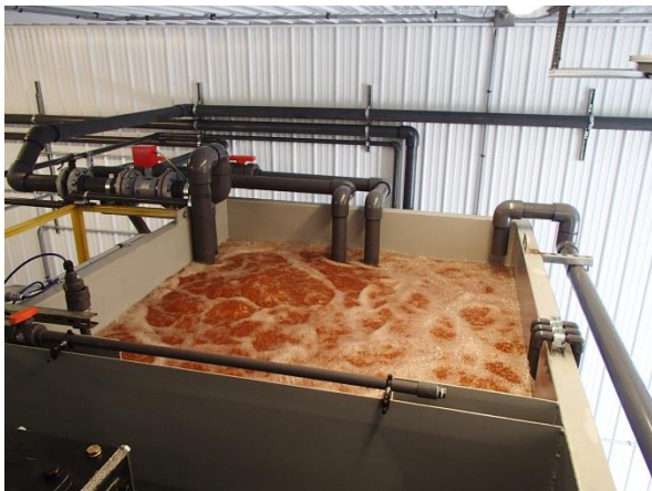
Raw well water entering treatment system
