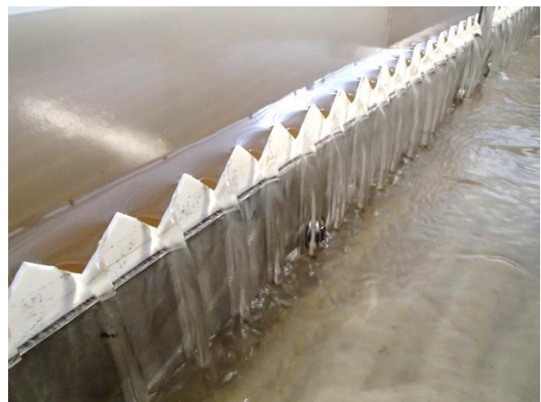
Treated water flowing over the effluent weir
