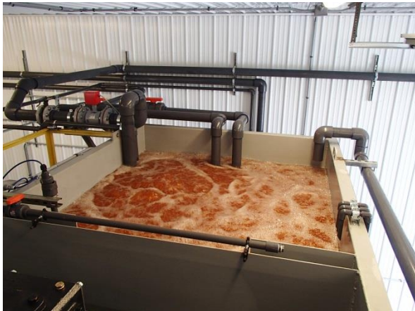
Raw well water entering treatment system
